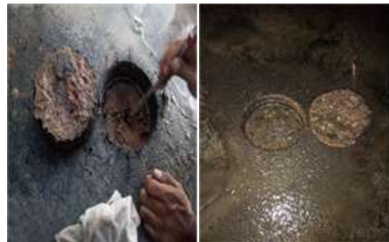
Figure 18. Soil under cracked hump shape pavement layer.
