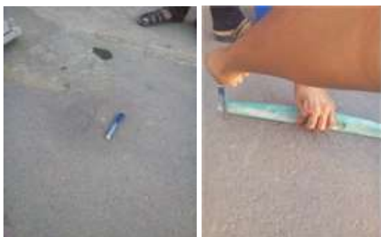
Figure 16. Cracks after one year.
